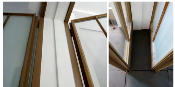
Fig. 12) Double Doors between the Hall and Dining Room. The measurements for both doors are different. The wall is the central point of the proportion.
